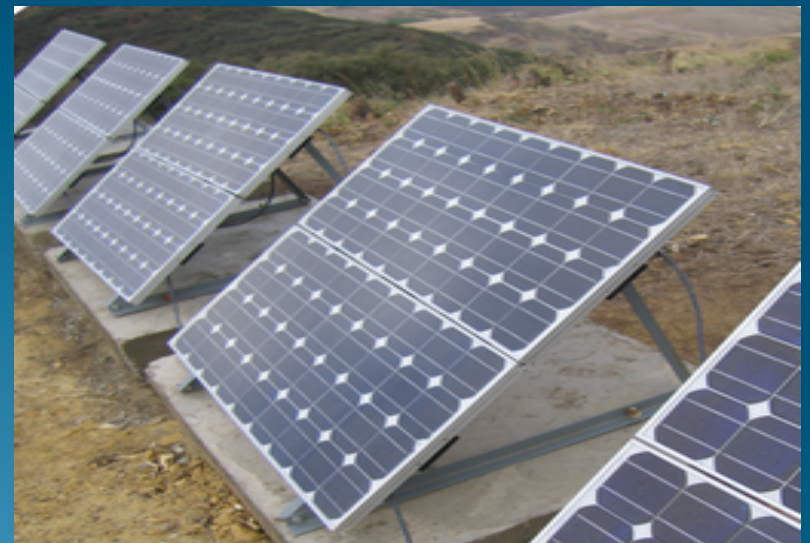
DC Power (Solar Panel)
